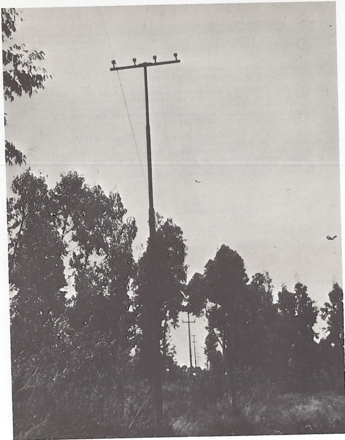
Figure V-74--Steel pole, 4-wire distribution line. Similar construction with modifications used at 15 and 45 kv., for Blue Nile River Basin studies.
